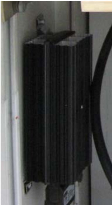
Heater Mounted in Cabinet
